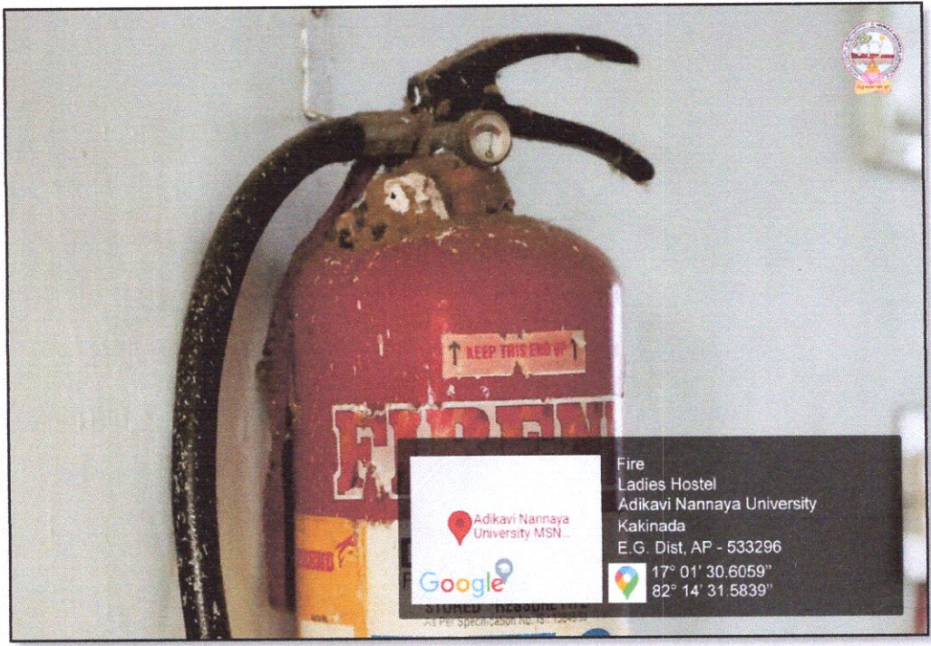
FIRE EXTINGUISHER AT LADIES HOSTEL,AKNU, RJY
